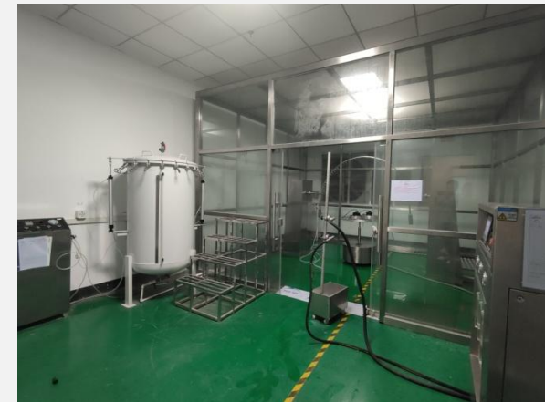
IPX Testing Room
